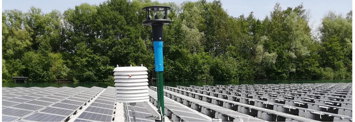
Measuring devices monitor wind and temperature at the Floating PV plant in Renchen, Germany.
